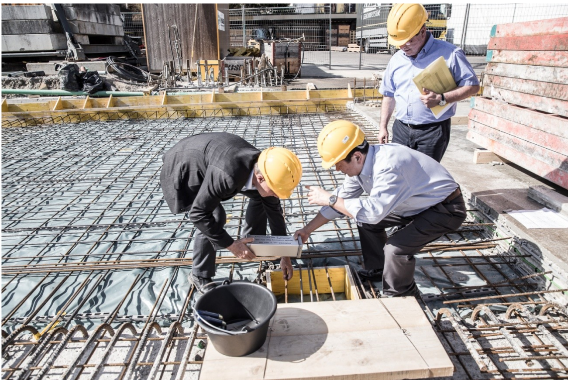
The foundation stone of the new building in Schwarzenburg is encased in concrete.
